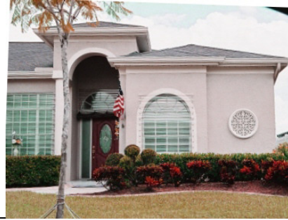
Unacceptable: plastic panels permanently attached to home.
