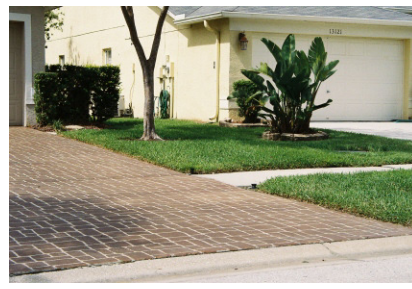
Unacceptable installation: paver material not flush with curb and street sidewalk. The paver material itself is acceptable.
