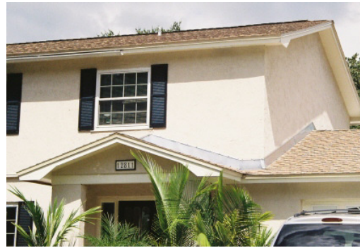
Unacceptable: unpainted flashing and roof drip edge
