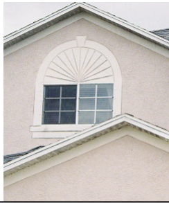
Acceptable: anchor bolts permanently attached to home
