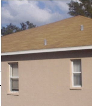
Unacceptable roofing: 20-year non-dimensional shingles. (Shingles are flat and have no shadow or thickness to them)
